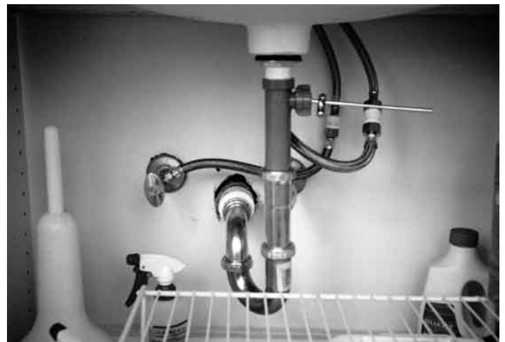
The new and beautiful plumbing installed by Irene.
